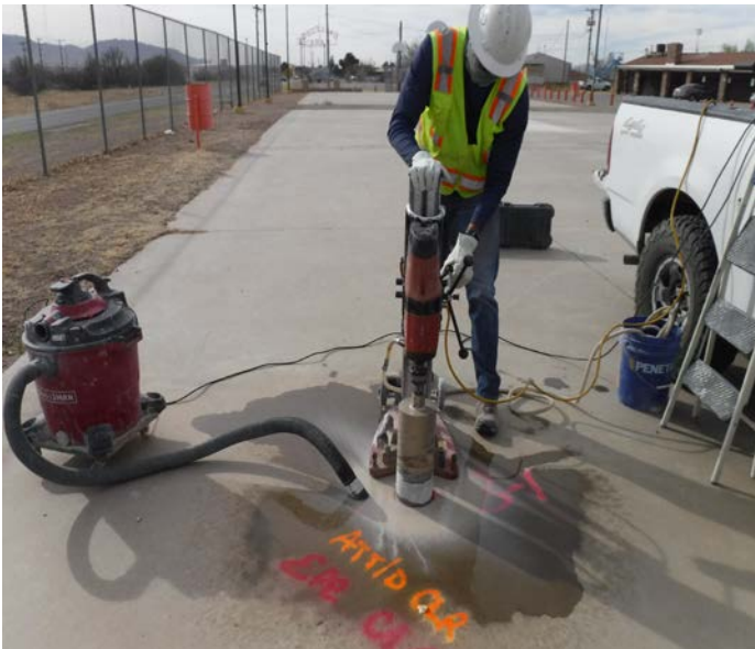
PHOTO NO. 11: General view of our coring operation at vertical boring B-5.
