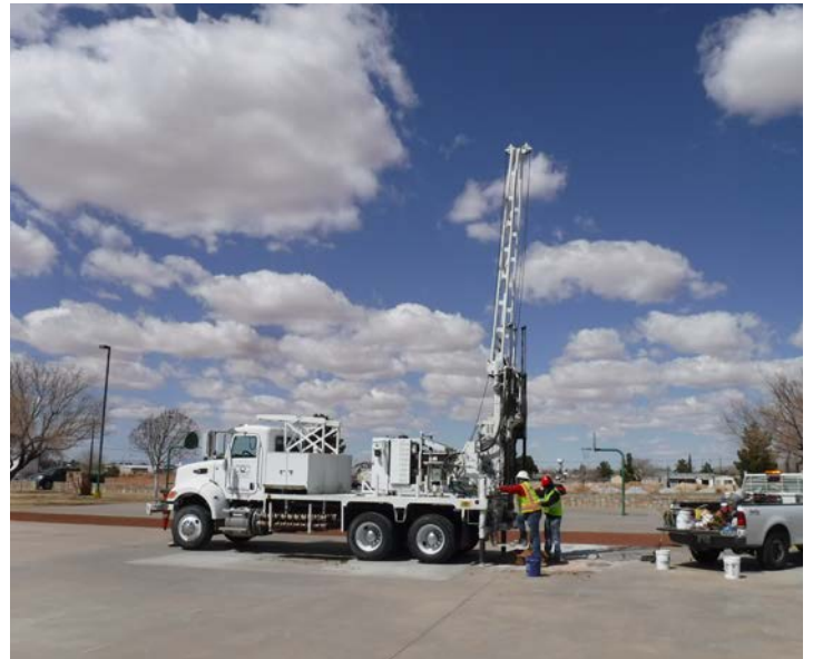
PHOTO NO. 4: General view of our subsurface soil drilling operations at vertical boring B-1. .
