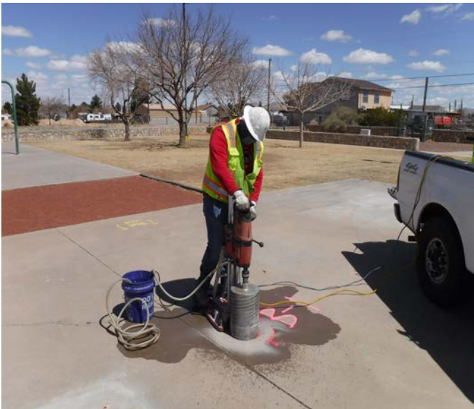
PHOTO NO. 3: General view of our coring operation at vertical boring B-1.
