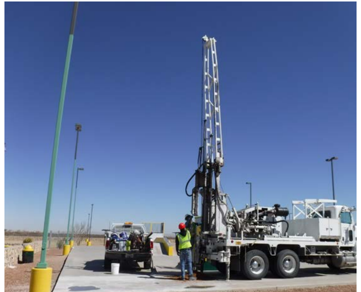
PHOTO NO. 8: General view of our subsurface soil drilling operations at vertical boring B-4.
