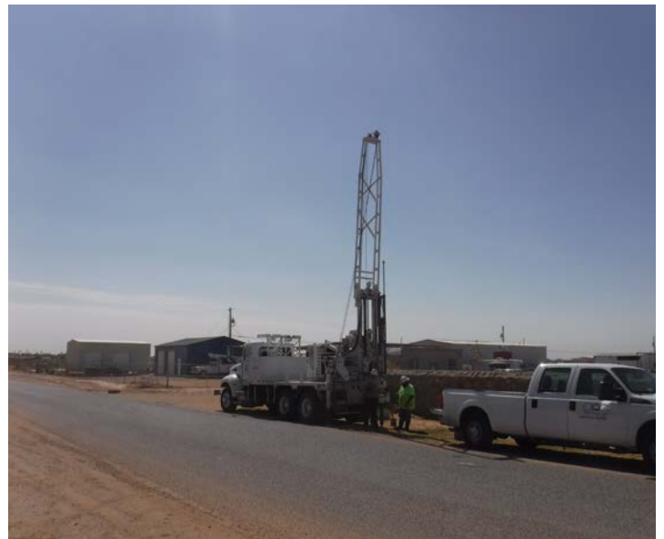
PHOTO NO. 12: General view of our subsurface soil drilling operations at vertical boring B-6.
