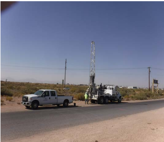
PHOTO NO. 11: General view of our subsurface soil drilling operations at vertical boring B-5.
