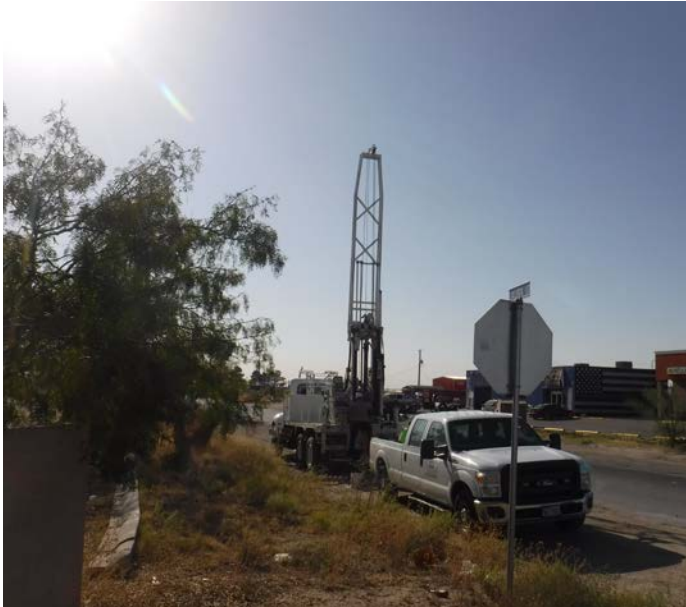
PHOTO NO. 9: General view of our subsurface soil drilling operations at vertical boring B-2.
