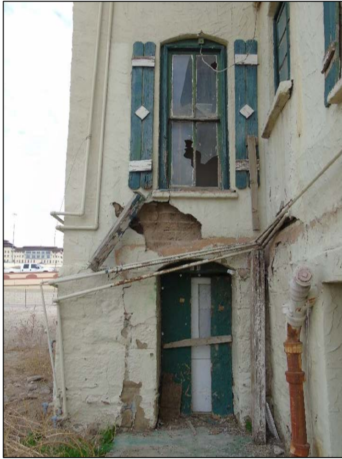
1836 West Paisano. Corner detail of north façade at “t” intersection, camera facing East.
