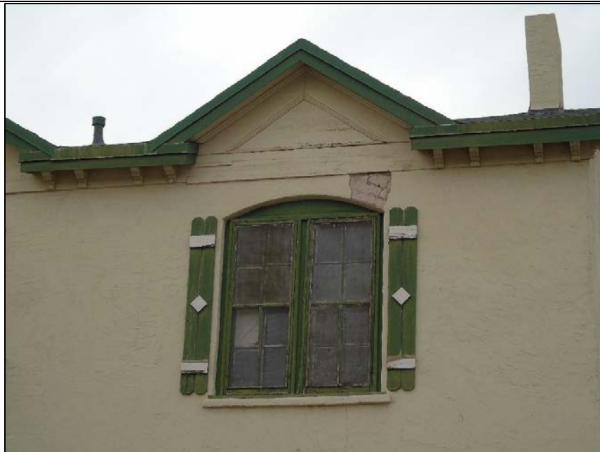
1836 West Paisano. Detail of brackets and window on front façade, camera facing West.
