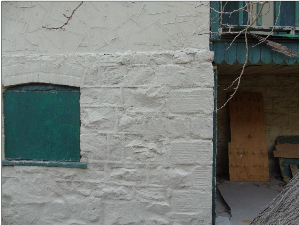
1844 West Paisano. Corner detail, north facade.
