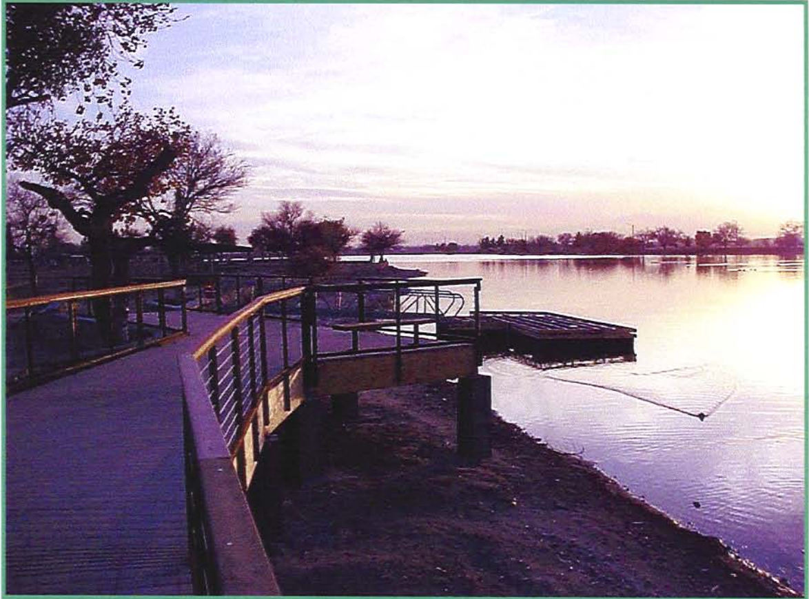
A view of a portion of the boardwalk and fishing pier improvements in progress on the Lake at Ascarate Regional Park.
